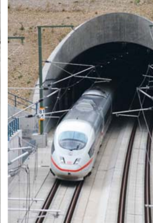
Overhead line fastening, Geisberg tunnel, Germany
